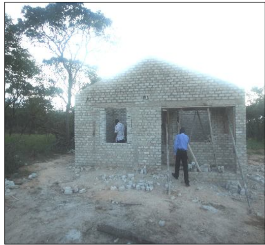
Fig. 14. 3 bedroom house under construction at the DMC "village" at ARDA Transau Estate.
