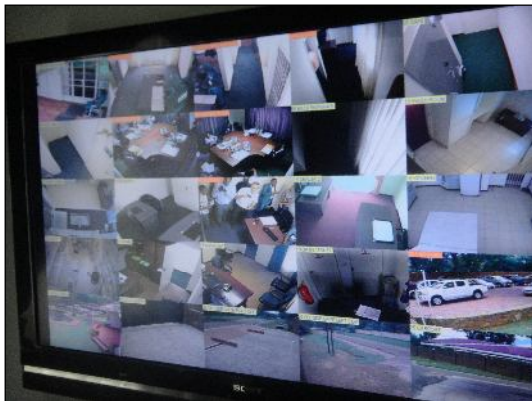
Fig. 12. CCTV-control room at the DMC Sorthouse.
