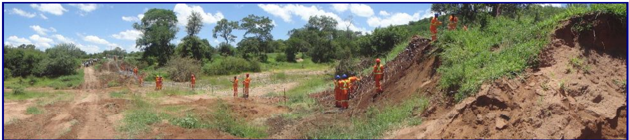
Fig. 11. DMC's "fence team" putting up the Pink Zone's security fence in the riverbed of the Chimberero River after torrential rains. As the image (taken on 6 January 2012) shows, only a few days after the heavy rains, the riverbed has almost dried out completely, providing a perfect pathway for intruders. Watchtowers with floodlights on either side, provide additional security.
